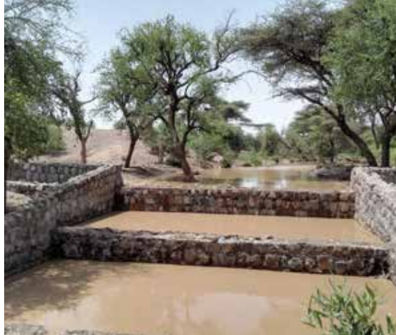
A completed water-spreading weir structure, showcasing its ability to slow floodwaters, recharge groundwater, and prevent soil erosion.
