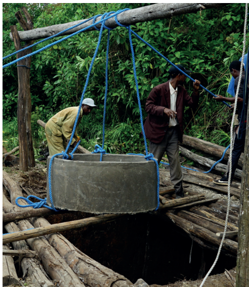
Well-building for solar water pumps to provide efficient irrigation.
